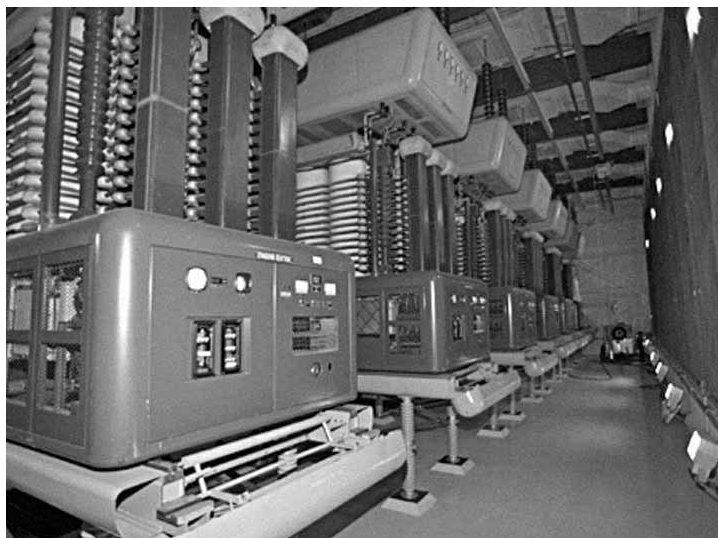
A view of the largest mercury arc rectifier ever built – this type of valve was originally used in the AC-DC conversion stations in the Nelson River DC transmission system. Most of these valves have now been replaced by thyristors. (Source: Manitoba Hydro).
