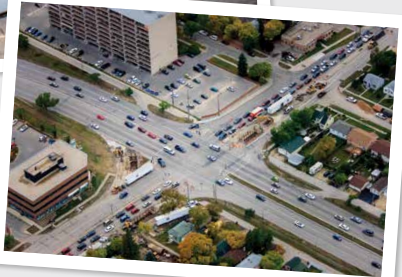
Ness & Century - Aerial View - construction at the intersection of Ness & Century. Ben Jablonski, EIT
