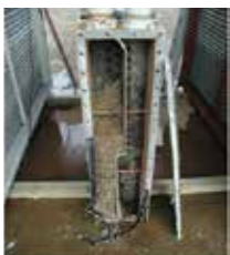
Figure 1: A cooler unit from Ontario Power Generation infested by zebra mussels. (Source: Ontario Power Generation)
