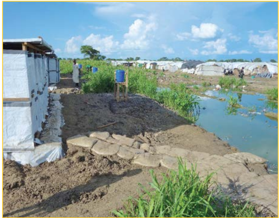
MSF constructed latrines and hand washing points in the Bentiu POC Camp
