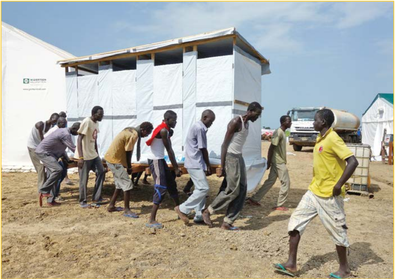
Moving a latrine superstructure in the MSF health centre in the Bentiu POC Camp
